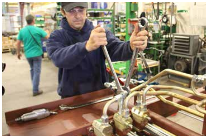
•At Check Valve end, loosen fitting connecting the Front of Cylinder #3 to Control Valve using 1-1/8" wrench and a 1-1/4" wrench.
